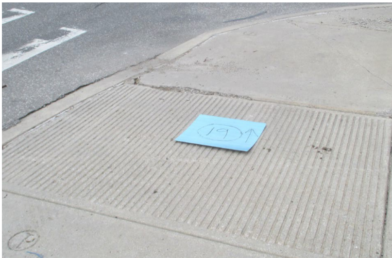
Picture 5: Deteriorated Sidewalks
