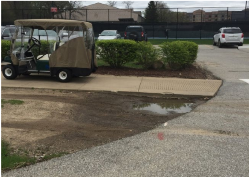
Picture 5: Level Changes Adjacent to Sidewalk
