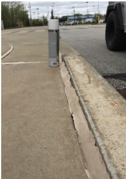
Picture 4: Level Changes at Curb-to-Sidewalk
